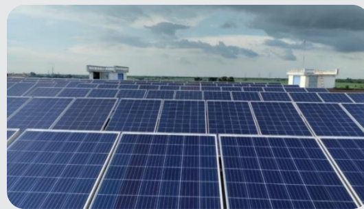
Figure 1: Rooftop solar PV system
